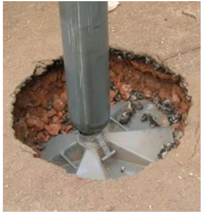
Example of an outrigger foot without a spreader plate (ground shear).
