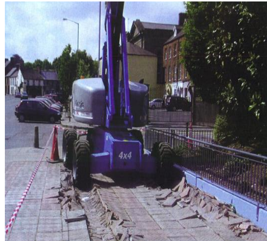
'Unsuitable ground conditions for selected MEWP'
