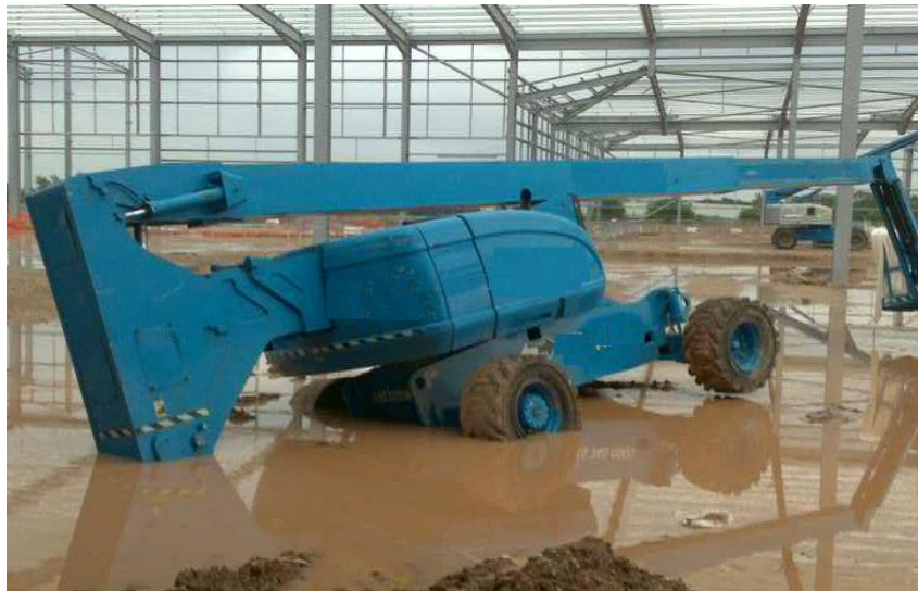
'Example of unsuitable ground conditions'
